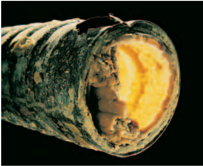
Figure 10-9 Dissolved minerals can build up thick deposits in plumbing pipes.
